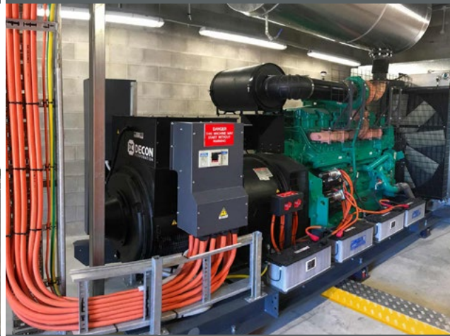
AUSTRALIA 2 X BASE FRAME 825/750 kVA
