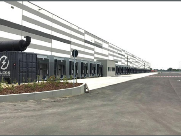
GDO LOGISTIC CENTER - PAVIA (IT) SS SUPER SILENT 1540/1400 kVA
