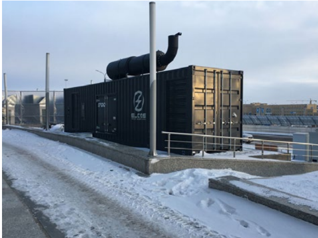
KAZAKHSTAN GENSET IN CONTAINER 40'1880/1700 kVA
