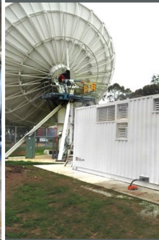
AUSTRALIA SATELLITE PLANT 2 X GENSETS IN CONTAINER 20
