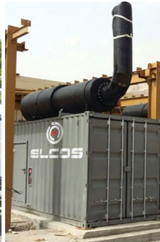
FAR EAST POWER PLANT 3 X GENSETS IN CONTAINER 20
