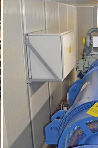
GS WITH NO BREAK DOWN IN CONTAINER
